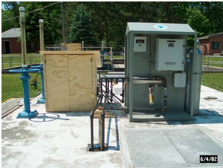
Example of Butane Injector 2000™ at a small wastewater treatment facility
