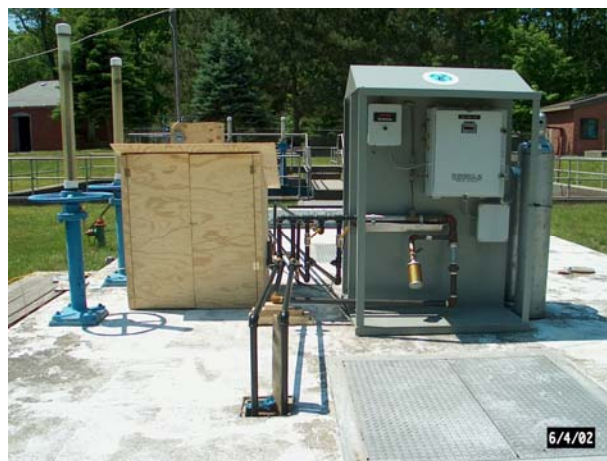
Example of Alkane (Butane) Injection at a small wastewater treatment facility
