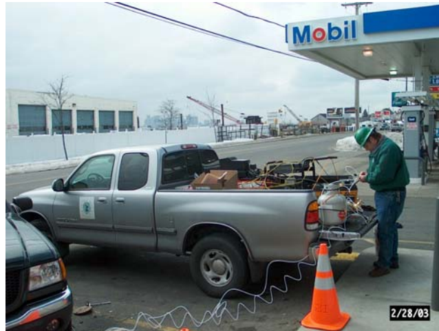
GBI personnel conducting hot-spot treatment using a Portable Butane Treatment System at an independent Mobil retailer located in Winthrop, Massachusetts
